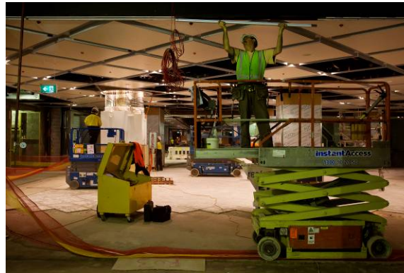
Photo: A worker installs ceiling finishes on Level 3 of the Westfield Sydney retail precinct.
